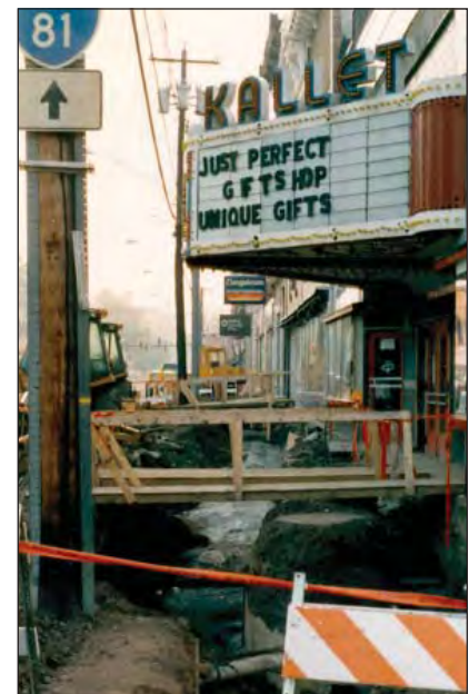
The burial of utility lines along Jefferson Street in the Historic District in Pulaski, 1989 (photo courtesy of Shawn Doyle).
