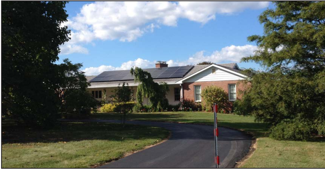
Solar PV array on Owasco home
